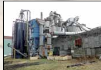
Industrial Wood Hog, dust collection and chip storage silos
